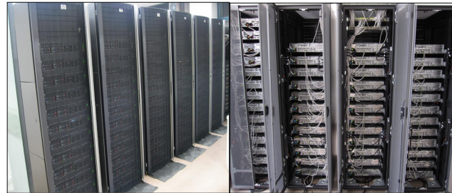
Data Center Front Side
